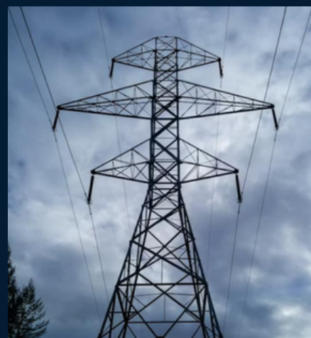
Power Utility Infrastructure
